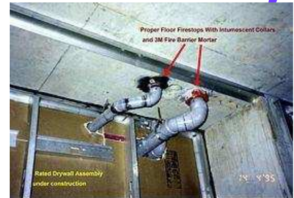
Northown Casitas, North York (now Toronto), Ontario, Canada, April 1999: Set-up for subsequent code infraction in plastic pipe wall penetrations: Improper hole sizing. Firestops (in the walls) the plumber considered to be the drywaller's responsibility. Floor openings are properly done in this case, with intumescent pipe collars and firestop mortar. The intumescent will expand and choke off the melting pipes. Drywall mud does not work as a plastic pipe firestop in the wall.
